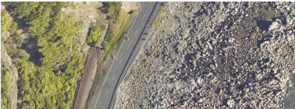
Figure 4 – Aerial imagery captured for NZ Transport Agency by AAM following the 2016 Kaikōura Earthquake identifies the rail track displacement and land uplift in the tidal area.
