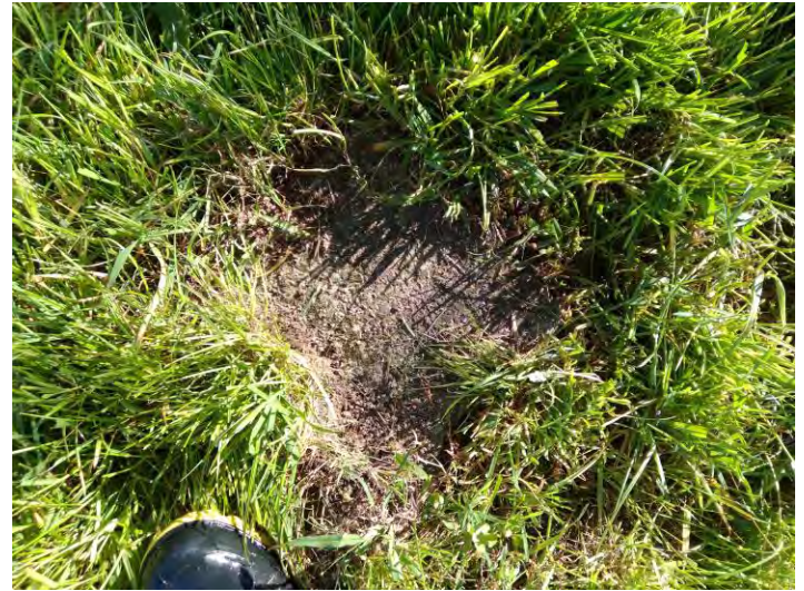
B4 – cement block protruding
