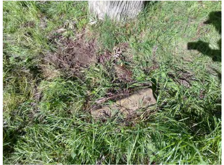
D4 – concrete block protruding
