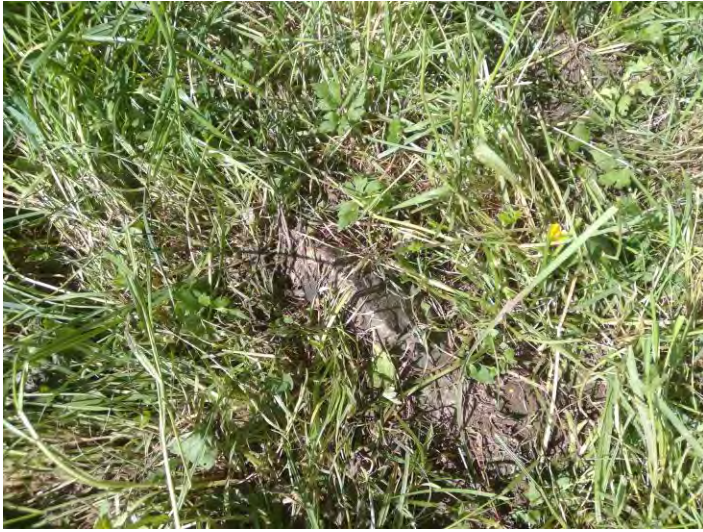
E4 – concrete protrusion
