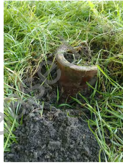
B3 – Ceramic pipe protrusion
