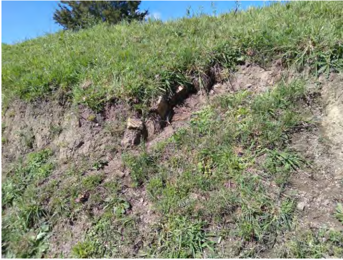
H6 – debris protruding
