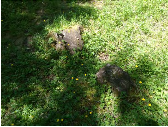
L5 – concrete protrusion
