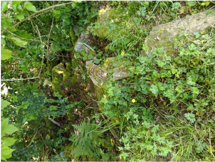
M6 – concrete debris
