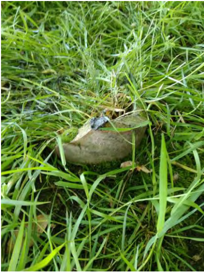
B3 – Ceramic pipe protrusion
