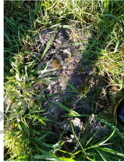
B4 – cement block protruding
