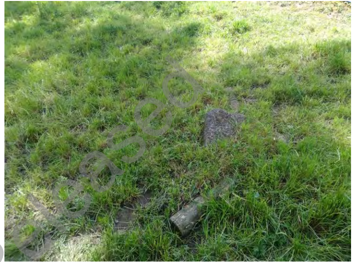
H7 – debris protruding
