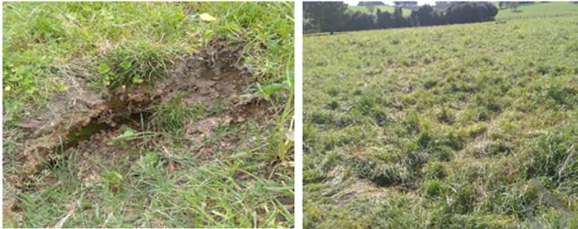
Figure 10: Instances of subsidence visible on site at areas E and A respectively (Left N7, Right E4)
