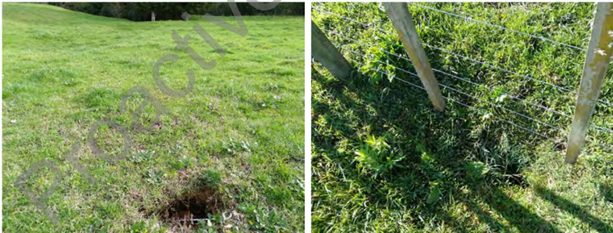
Figure 9: Evidence of damage to landfill cap in Area E and at extent of Area A (Left N7, Right A3)
